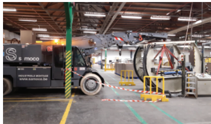
Installing a cardboard turner at Van Genechten Packaging with our Ormig Electrical crane
